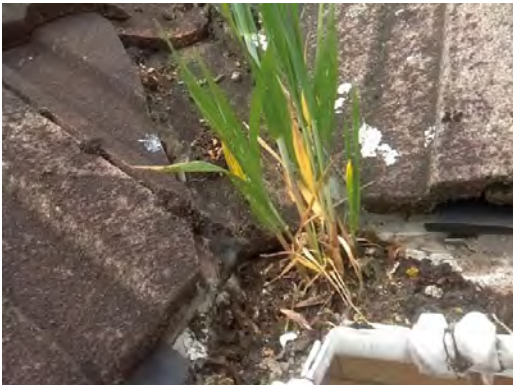
▲ The culprit causing the rainwater to spill over
